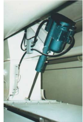
Silo feeding installation for belt conveyor system
