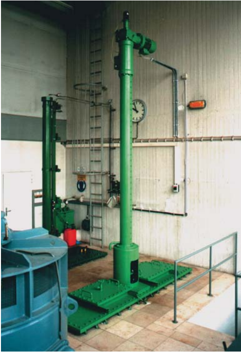
Flood gate actuator
