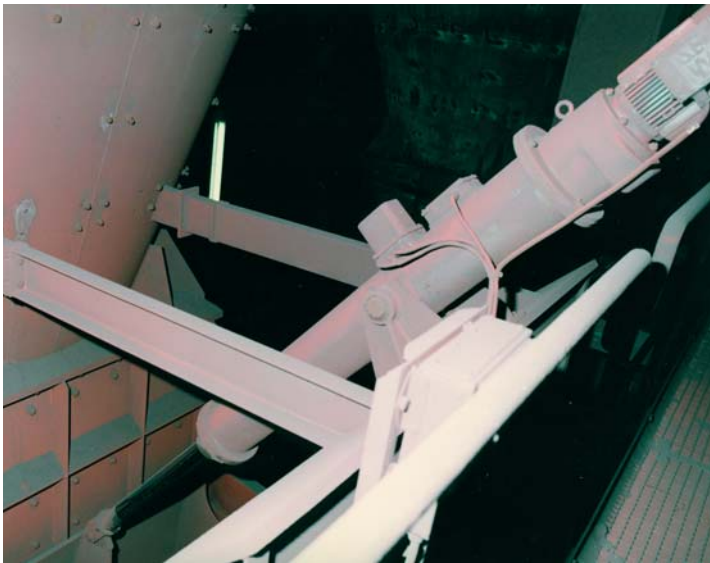
Bunker flap control in steel plant
