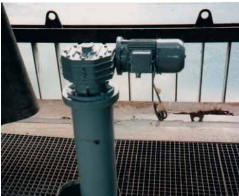
Flood gate actuator
