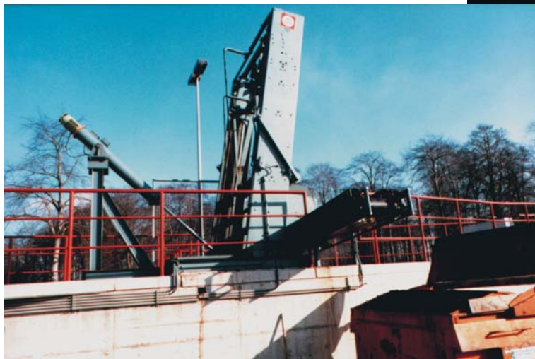
Clarification plant Actuator for rake control
